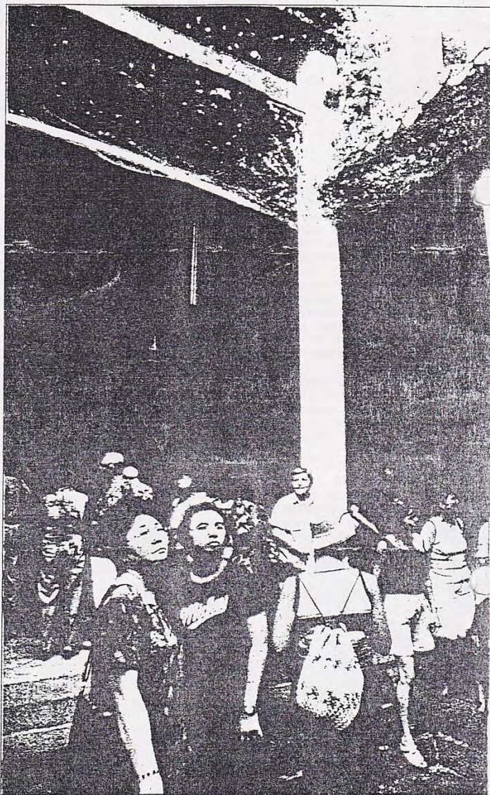
DILAPIDATED STATE... a sense of neglect and abandon mark the main hall of the Chung Keng Kwee ancestral temple. - STARpix by LAWRENCE SEOW
